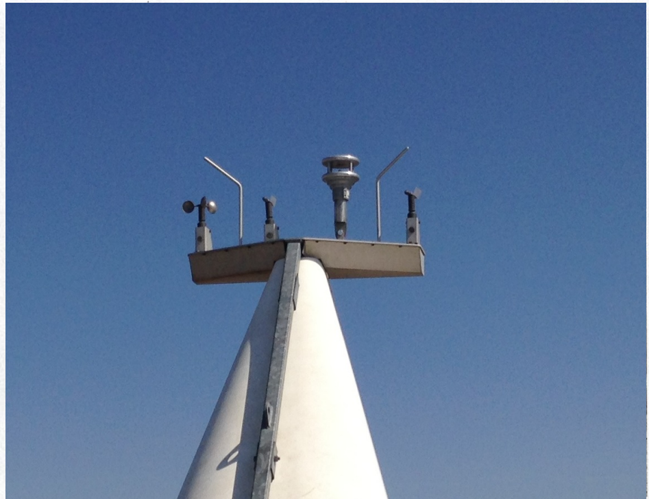
An ultrasonic sensor (the round dome) mounted on top of a turbine showed it could measure wind speed and direction more accurately than the OEM's mechanical anemometer and wind vane, providing vital information to the PLC.
