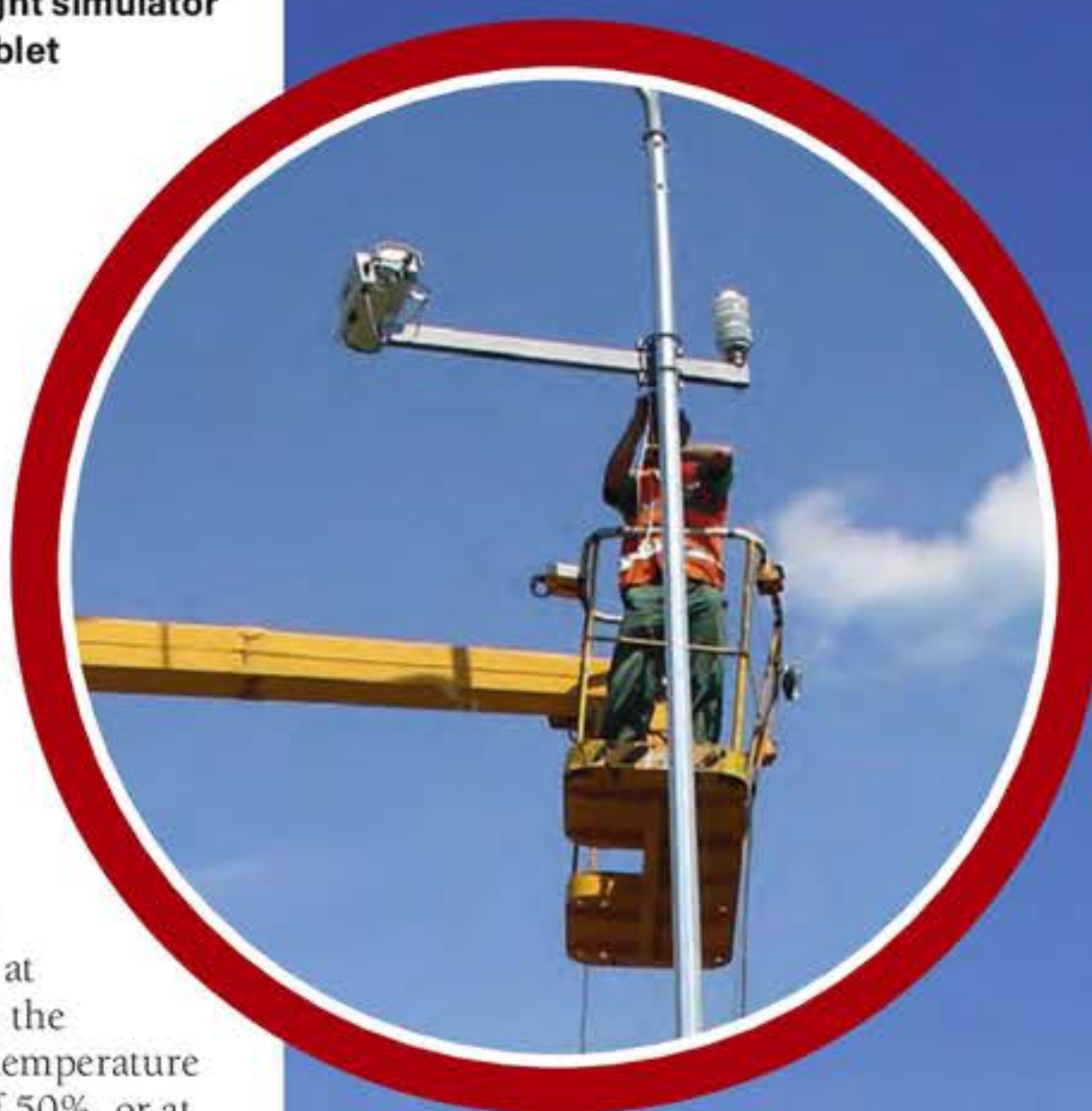
↑ On-site calibration at Albis Pass, Switzerland
