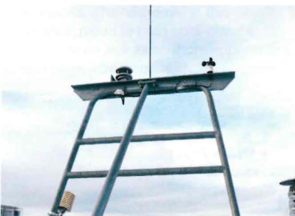
Wind Park in Rivière au Renard monitored by Lufft VENTUS ultrasonic wind sensor
